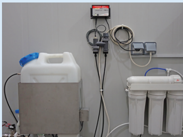
Water treatment systems
