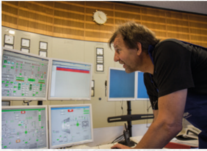
All the information is brought together in the control room of the Leitzach plants.
